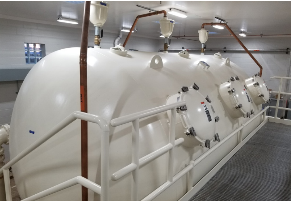
..... Below: Inside the well pumphouse on Locust Grove.
