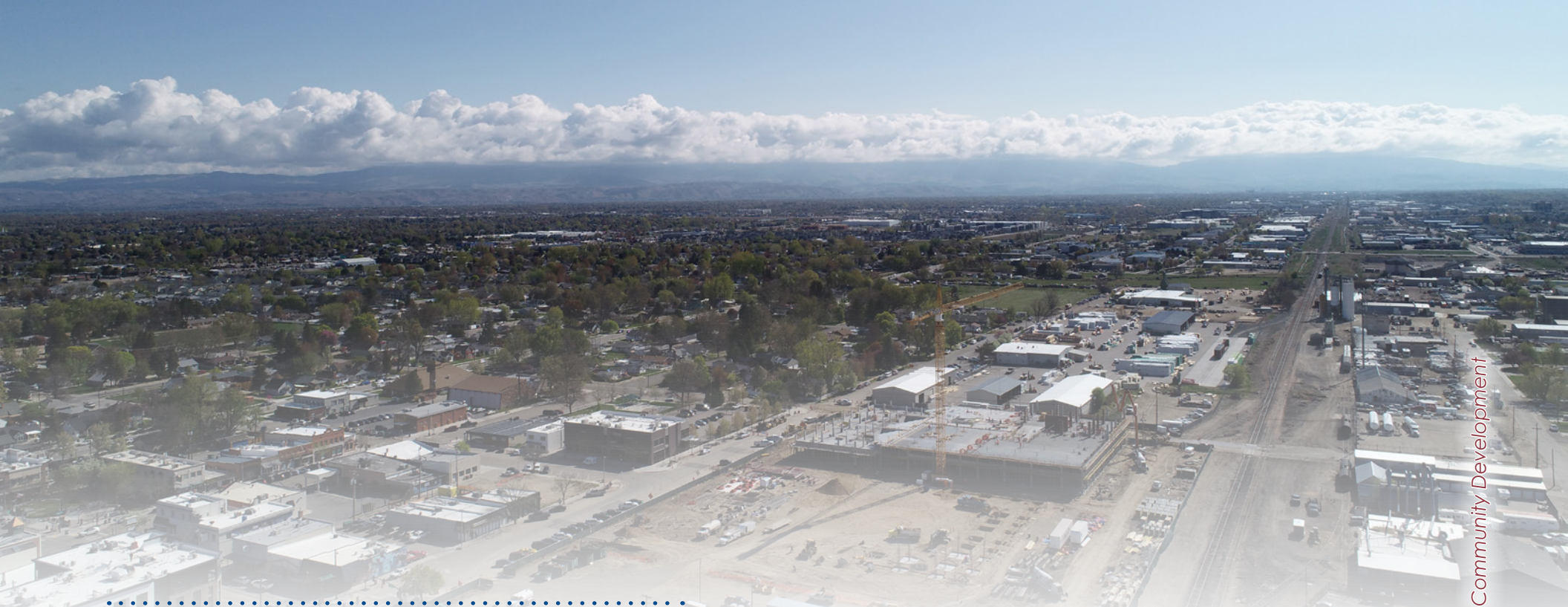
..... Above: Construction along the Boise Cutoff spur rail corridor, looking towards the north-east.
